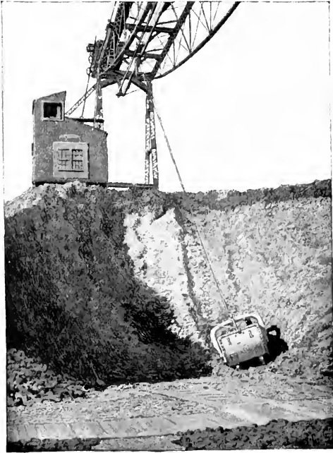
A Shovel-bucket in Use at the American-built Storage and Rehandling Plant at Mariupol, Russia.
